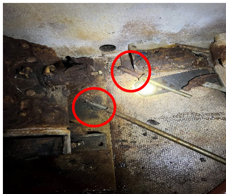
Figure 2. Broken cable guide Anne's Bait Shop Ingleside, TX. (February 20, 2024/USCG)
